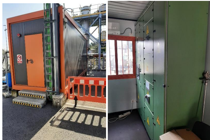
Figure 6: CASOH electrical room
