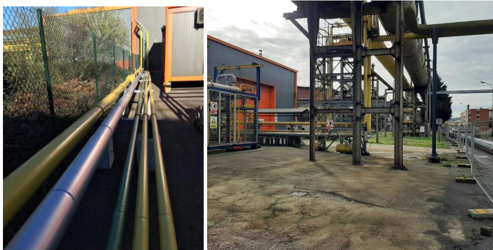
Figure 4. Utilities ring (left) and industrial gas pipelines connection to laboratory
