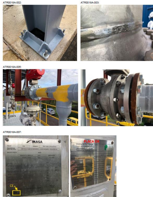
Figure 16: Images for points of improvement in the pilot plant
