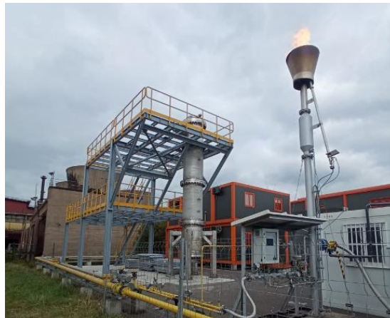
Figure 26: Off gas system tested with fuel gases during acceptance tests.
