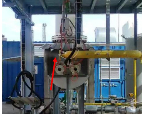
Figure 22: Example of a cleaning test, showing dust and debris coming out from the N2 line to the preheaters.
